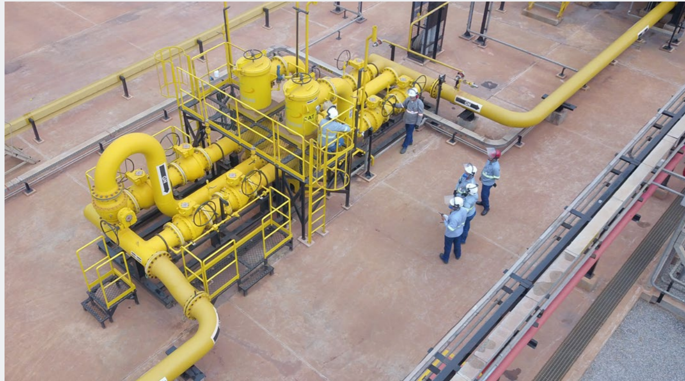
Natural gas installation at Alunorte.
